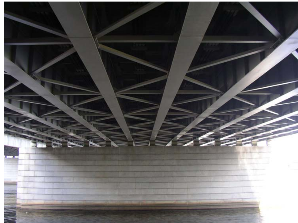
Photo 6 – Typical Pier and Superstructure of the Three Bridges over the Potomac Rive (Rochambeau Memorial Bridge Shown)
