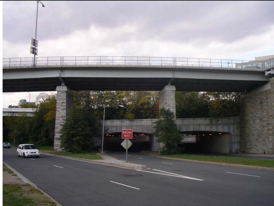
Photo 9 – East Elevation of the Ramp from I-395 Northbound to 12 th Street (Foreground).
